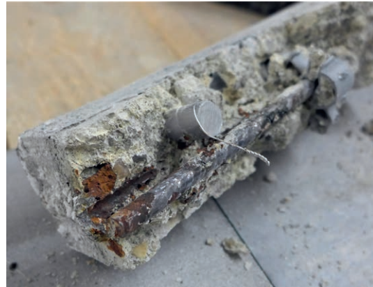
Figure 11: Typical contact point between stainless steel rod and corroded B500 reinforcing steel, low local, only surface corrosion on stainless steel | photo: Jürgen Triebert
