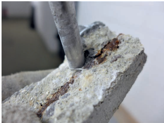
Figure 10: Refurbishment variant B after breaking the test specimen; the carbonated normal strength RC can be seen after removing of Pagel TF 10 layer; typical picture with very strong corrosion on the unalloyed reinforcing steel B500, mostly over the entire circumference and the entire length | photo: Jürgen Triebert
